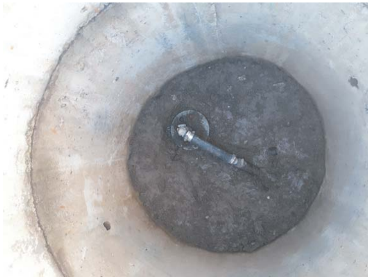
Photo A (above): Wellhead of W-2
