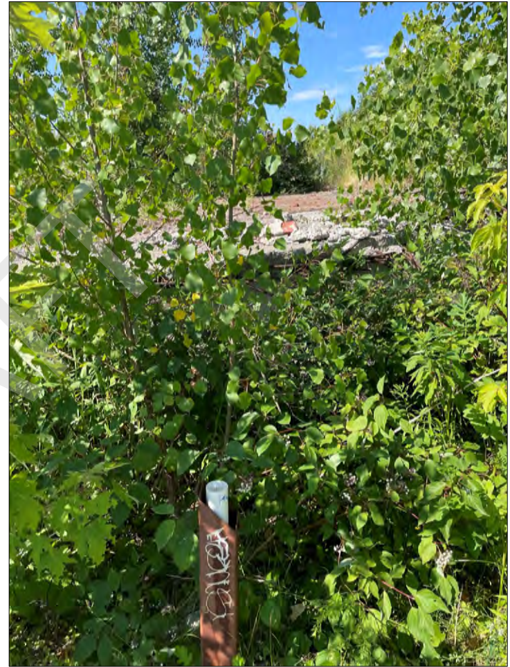
Photo 2 – Damage well casing looking South located in front of old building foundation – MW80. July 11, 2022
