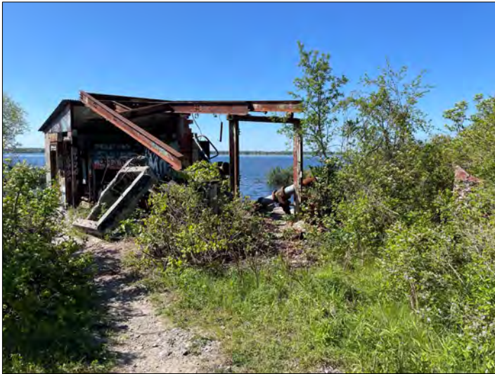
Photo 9 – Old pump house looking South at the southern tip of the Peninsula lands. May 26, 2023.
