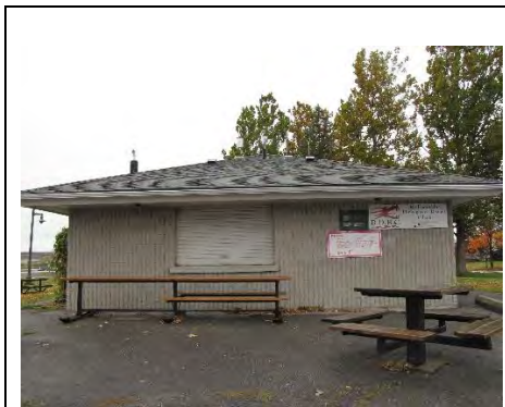
Shingle roofing shows some signs of wear
